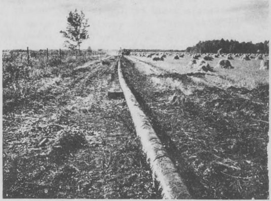
18 While farmers worked their fields nearby the pipe line progressed without interfering with the harvest. Each farmer received payment for right of way and for any loss of crop
